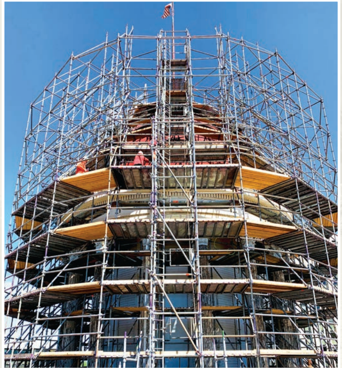
Restoration of both the interior and exterior of the Old State Capitol dome is projected to be complete by late fall.
