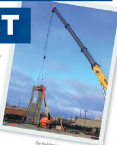
The building started to take shape once the precast walls were installed.
