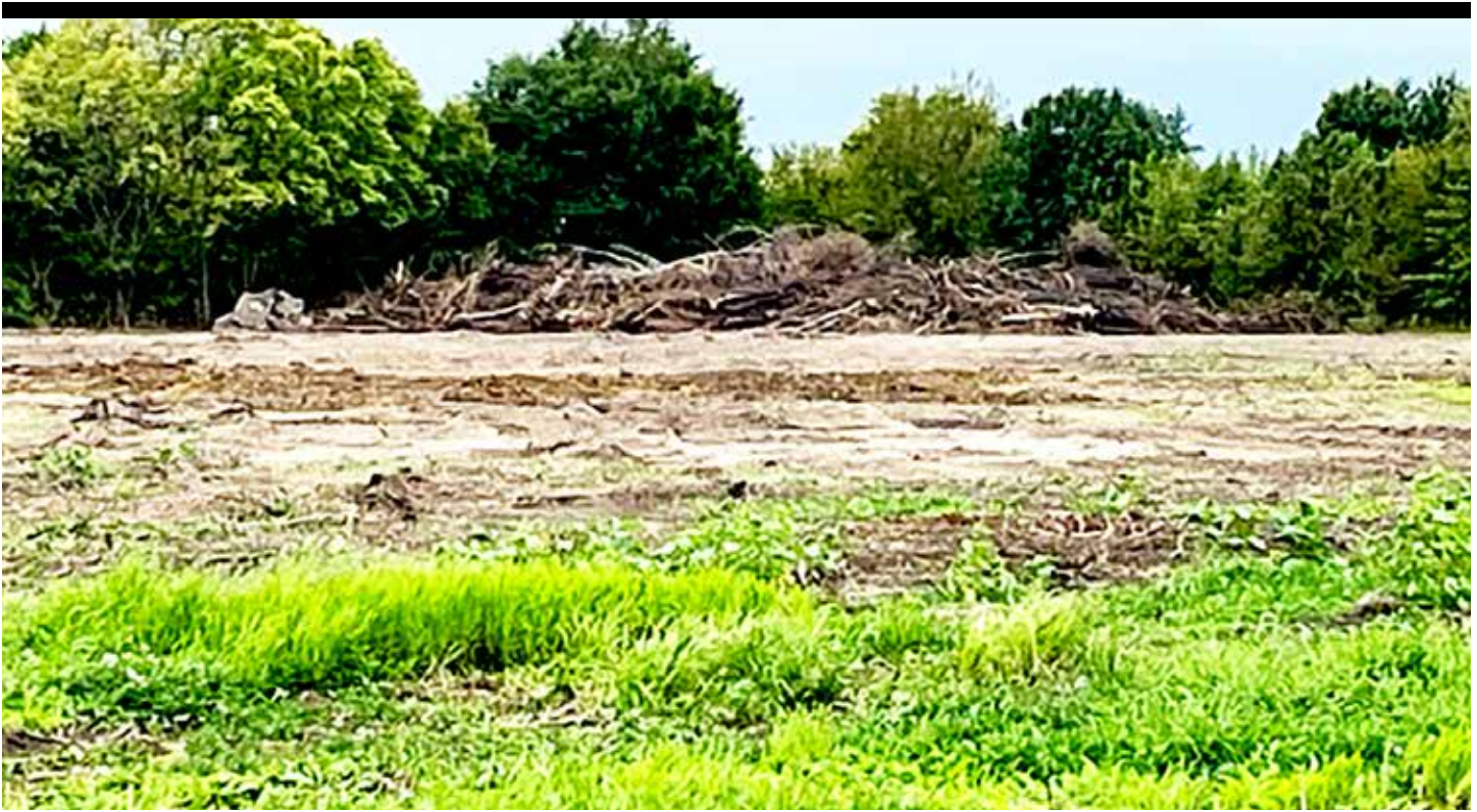
Joyner Construction Services is clearing land in the 3100-3200 blocks of Mercantile Drive in preparation for construction of a new apartment complex on the west side. PHOTO BY DARON WALKER
